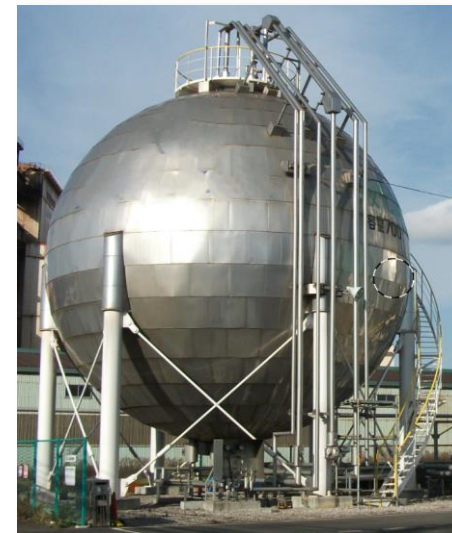
Currently constructing a total of three spherical tanks for liquefied carbon dioxide.
