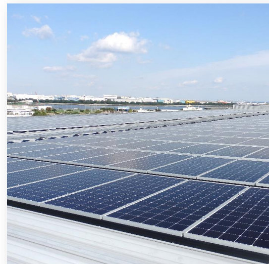
Higashi-Kojiya Fourth Power Plant
