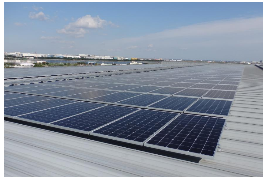
The Company's first project subsidized by the Tokyo Metropolitan Government (Higashi-Kojiya Fourth Power Plant)
