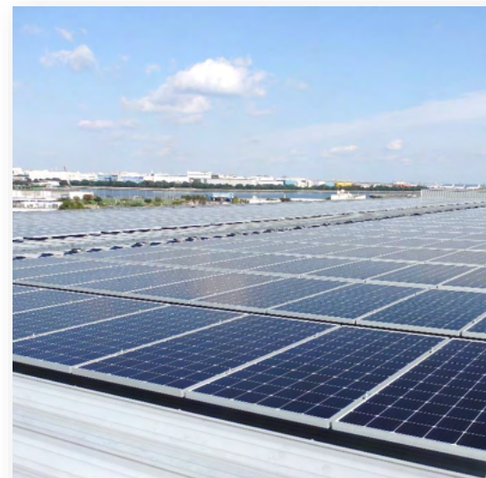
Higashi-Kojiya Fourth Power Plant
